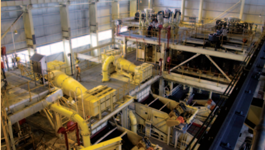
Interior of the preparation plant
